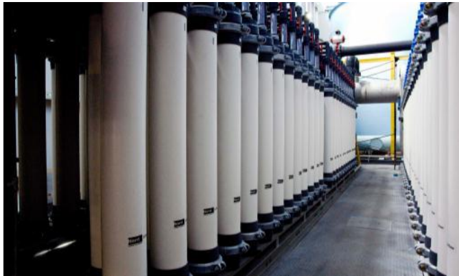
POTABLE WATER TREATMENT Keokuk Water Works – USA 1,500 m 3 /h
