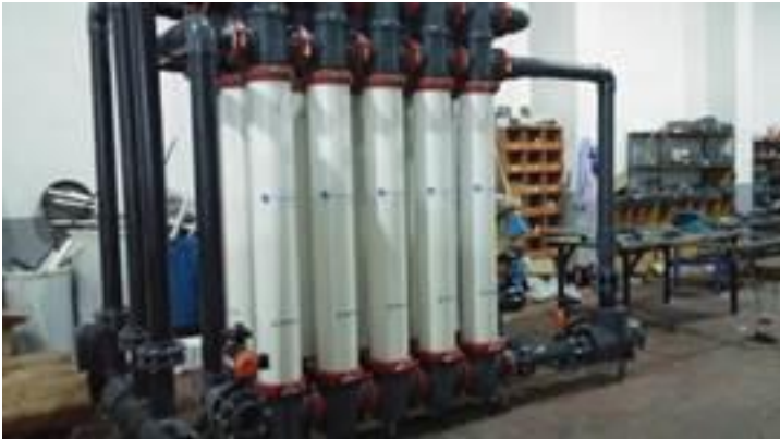
PROCESS WATER TREATMENT TKI – Ankara (Turkey) 70 m 3 /h
